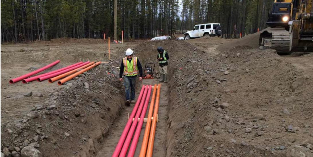
Note: Trench width to allow safe worker access, trench top edges pulled away, conduits properly spaced
