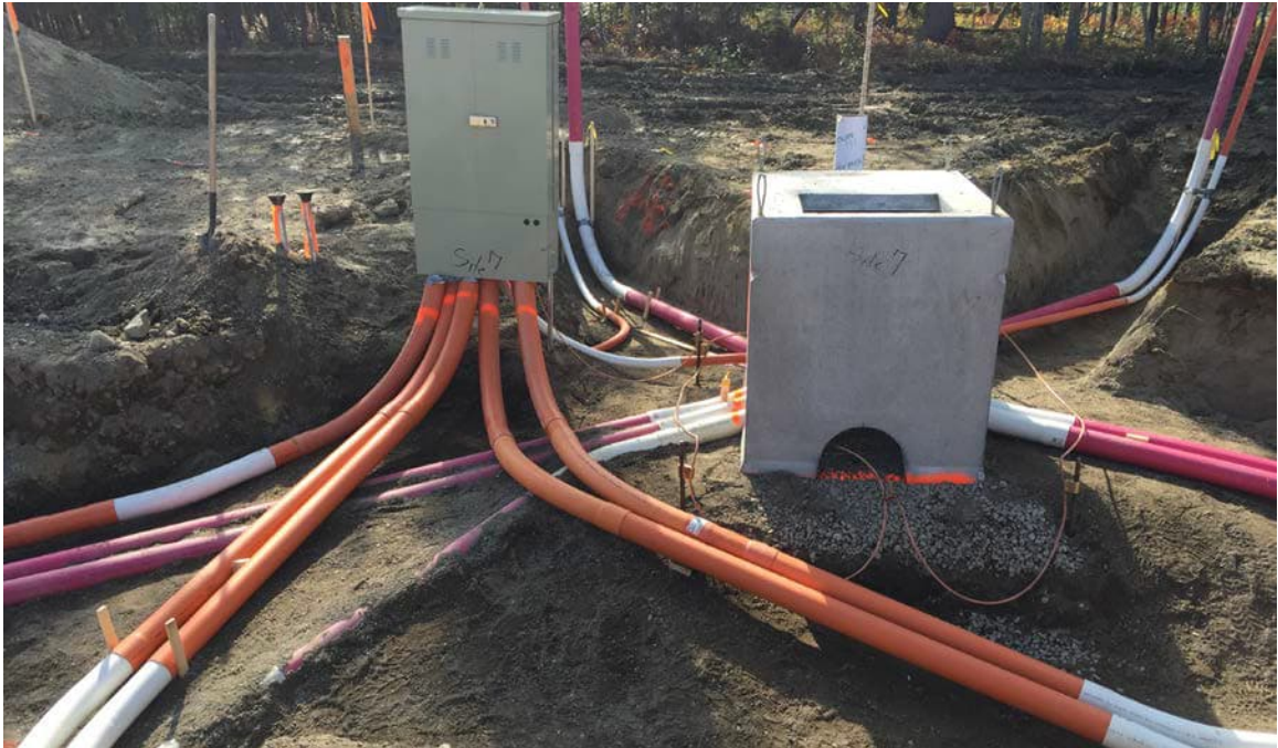
Note: Both photos show communications conduits do not pass through the ground grid.
